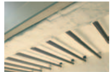
Heating elements in furnace hood
