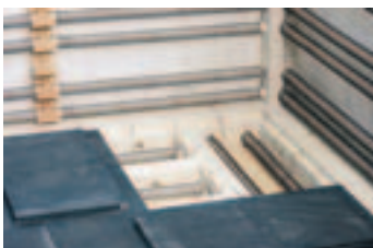
Tub heating elements covered by SiC tiles to create level stacking support
